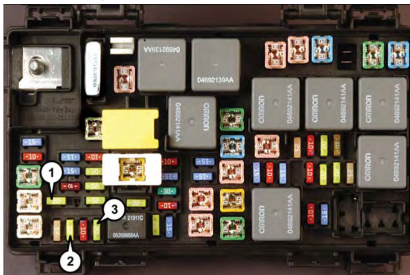
Power Outlet Fuses
