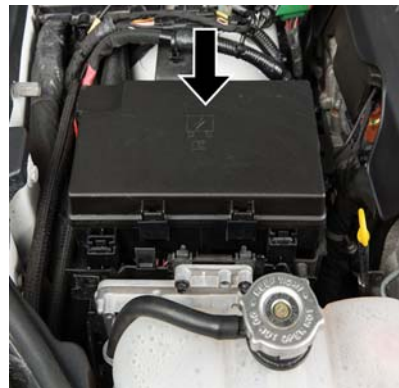
Power Distribution Center
