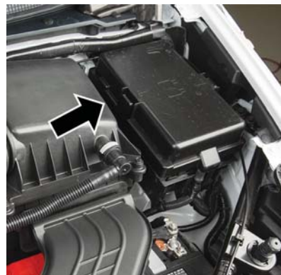
Power Distribution Center
